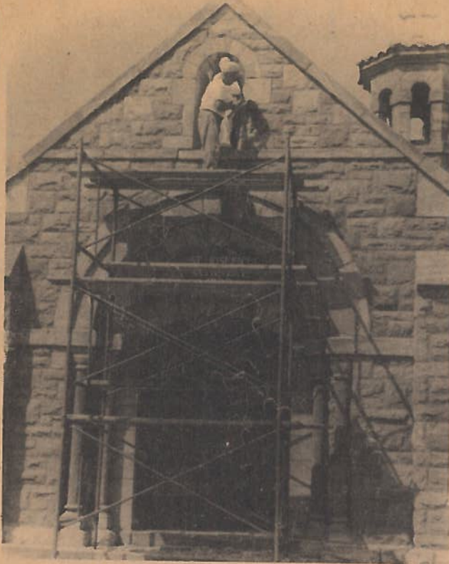
Angelo Manella restoring the facade of St. Joseph's Cemetery Chapel during this past summer. -Bob Gates photo Vol. V No. 46
