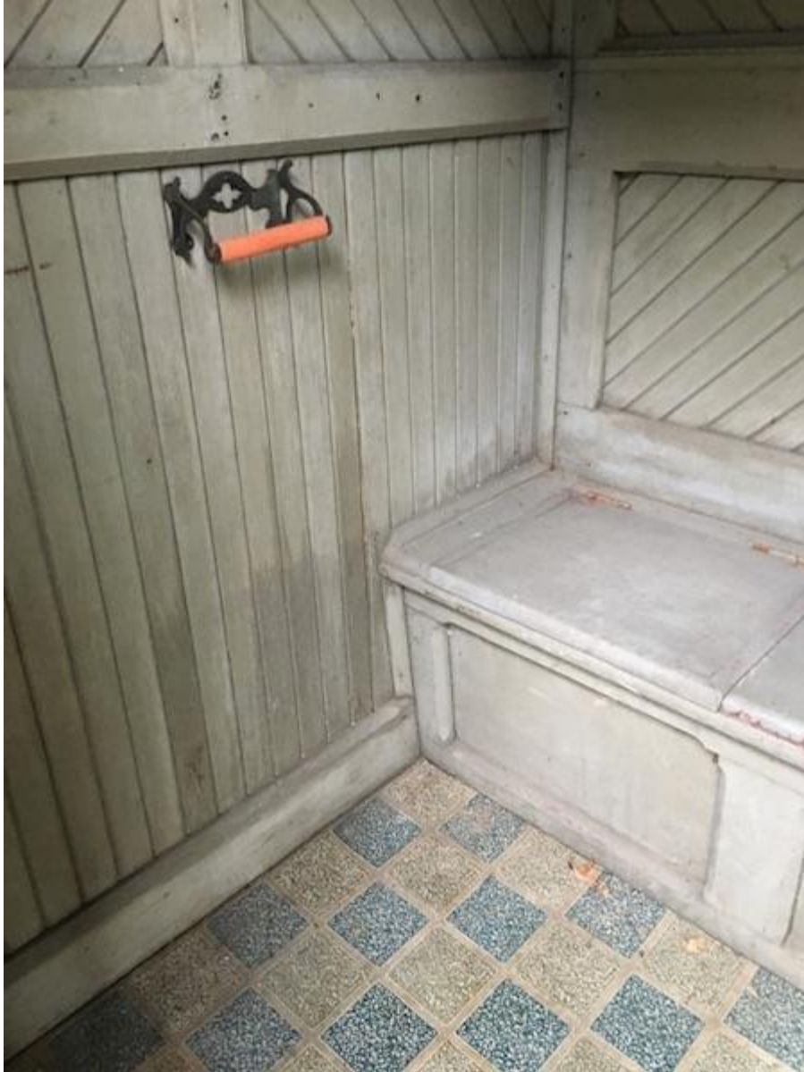
The high water mark for that flood is still visible inside the Eastlake outhouse located next to the Print Shop. The water line is just above the row of seats.
